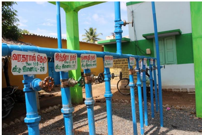
Photo 6 Water metres on the distribution network in Ramianahalli
