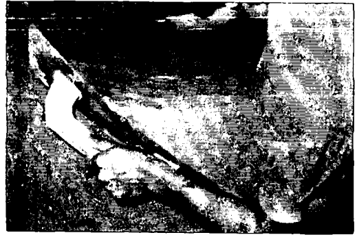
Fig. 8 Coating the surface of the core with well puddled clay using the float.
