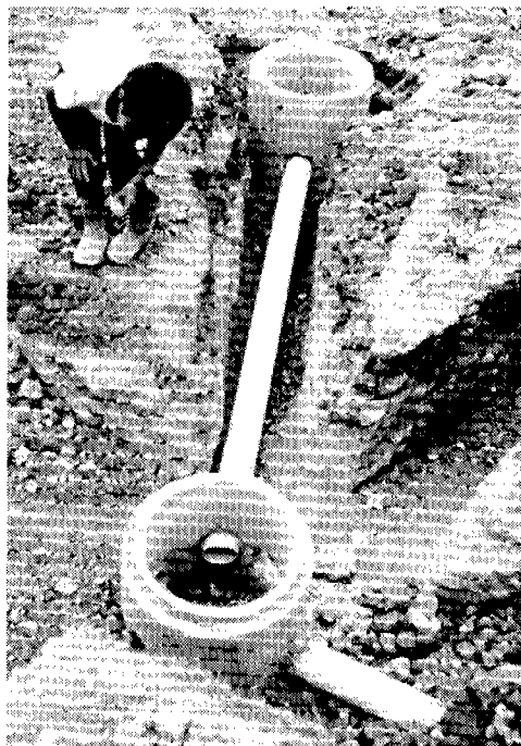
Figure 5.5 Junction chamber for simplified sewerage using larger diameter concrete pipes, used in Guatemala.
