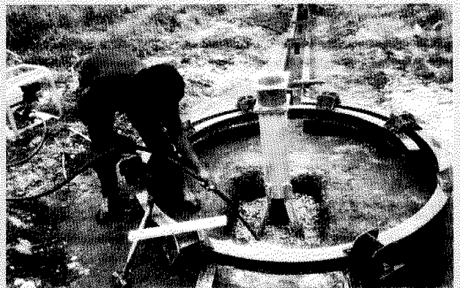
A worker prepares a concrete cast for the installation a borehole in Mpigi District under the JICA funded project
