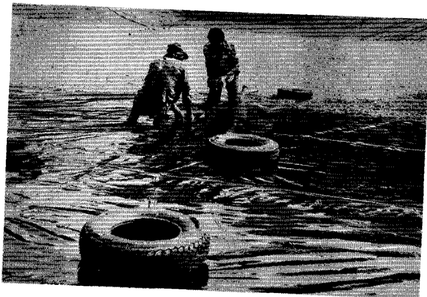
4. Sealing a joint in the black polyethylene sheet. Note limestone aggregate covering in background.
