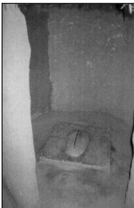
Better technical know-how among those who supervise latrine construction will mean better workmanship
