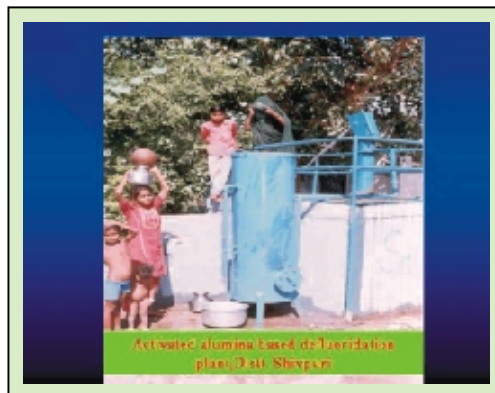
Fig. 1.1: Defluoridation plant in Madhya Pradesh
