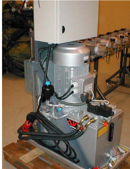
The new high-pressure pump
