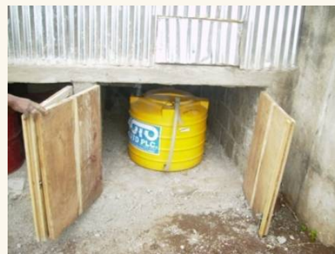
Figure 2: Urine storage in UDDT toilet
