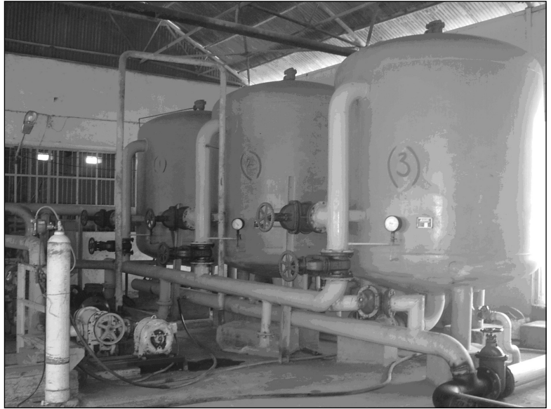
Pressure filter in towns in Gezira scheme
