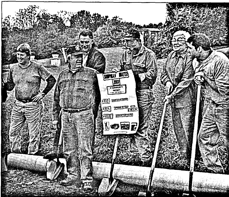
This photo shows the initial groundbreaking for the Shipman (Va.) project, whose objective via Self-Help Virginia was to eliminate the shortage of water to households served by the project. The project also addressed Shipman residents' complaints of irregular flow, discoloration, odor, taste, and the suspected presence of volatile organic contamination in their well water.
