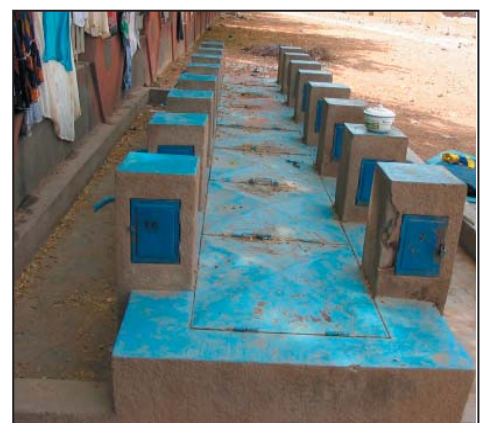
Water box taps in Burkina Faso
