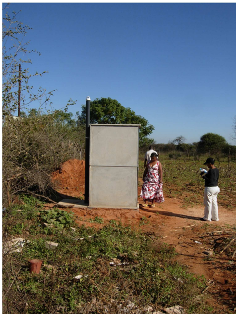
Figure 1 The eco-toilet model has a ventpipe against bad smells. Photo: Dick de Jong, IRC
