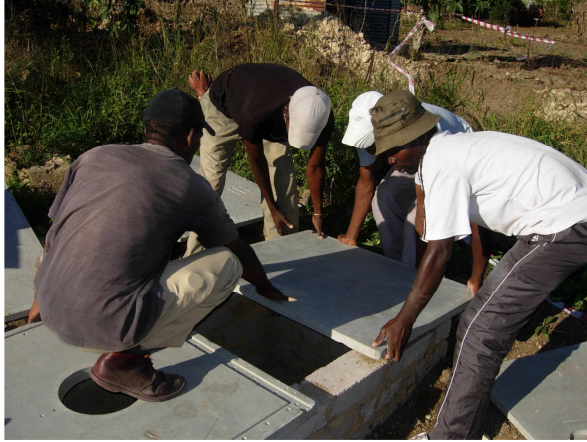
Figure 3 The pit under the slab is 2 meters deep. Photo: Dick de Jong, IRC
