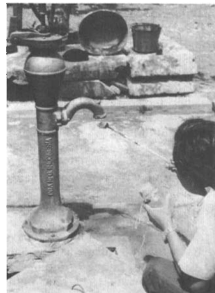
Sanitary worker sampling and inspecting converted dug-well with insanitary cover and handpump.
