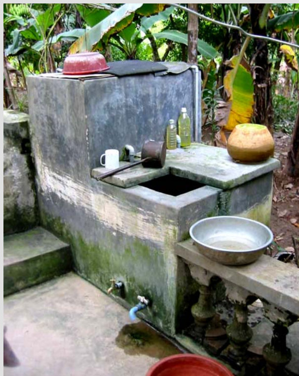
Sand filter on top of storage tank
