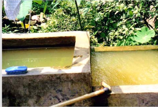
Settling tanks (right: tank 1 for aeration and settling; left: tank 2 for further settling)
