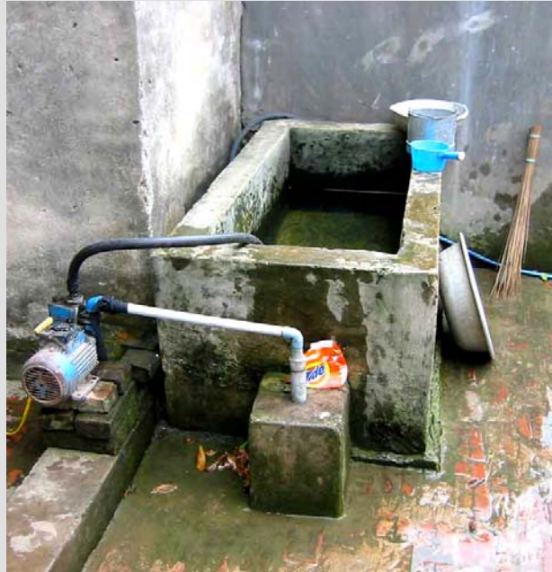
Electrical pump and storage tank
