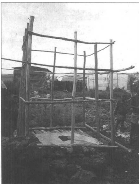
Family latrine construction. Some materials were provided by Oxfam; the family improved on the basic design with their own piece of sheeting.
