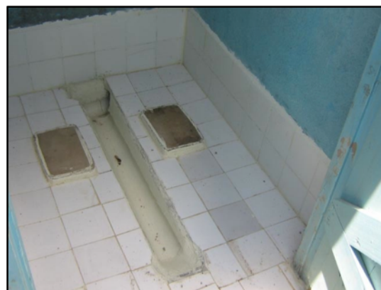
FIGURE 0. TILE FLOORING WAS USED FOR THE URINAL IN ATONO PRIMARY (PHOTO BY IMELDA AKINYI)
