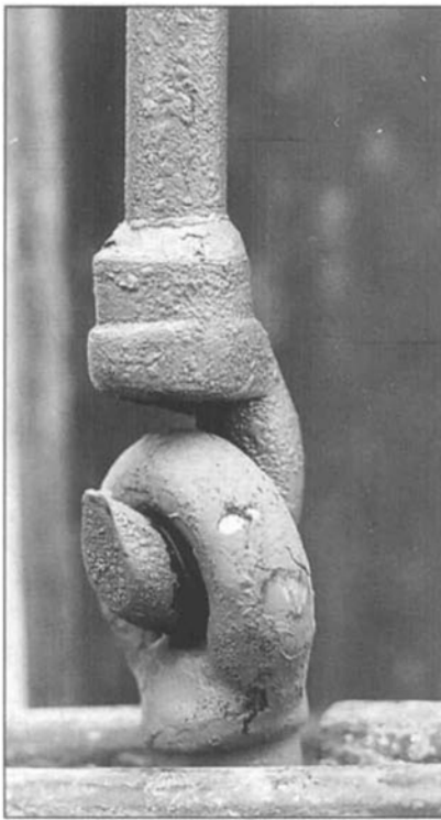
Close-up of hook-and-eye rod joint after 18 months' operating in aggressive water conditions at Idaho Farm.
