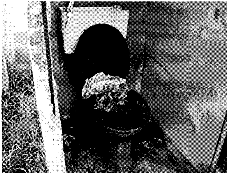
Figure 1 | Blocked flush toilet.
