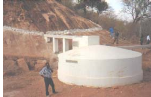
An aqueduct gravitating run-off water from a rock to a tank at Kibwezi.
