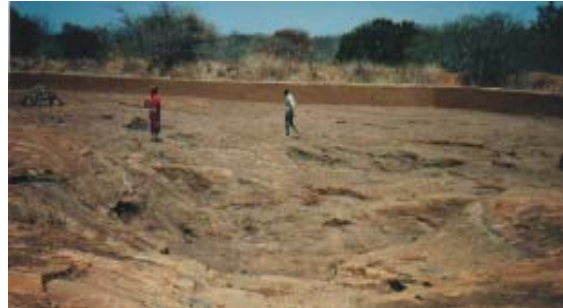
An underground rock was cleared of vegetation and soil in Mutomo. Deep rock pools were found where trees had grown. A low masonry wall was built along the lower side in 1985.
