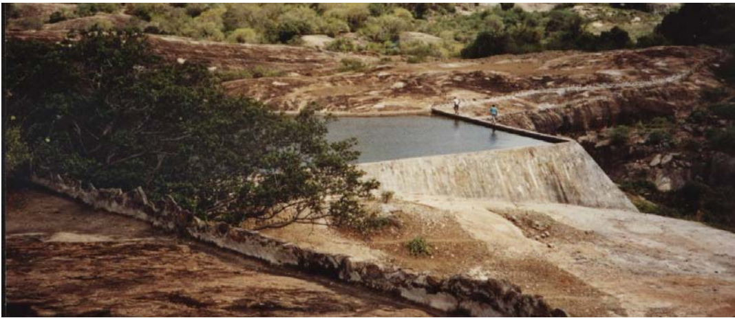
A masonry dam, Kaseva Rock Catchment Dam, built by ALDEV at Mutomo in Kitui in 1956. The two persons walking on the crest give an idea of the dimensions of the dam.
