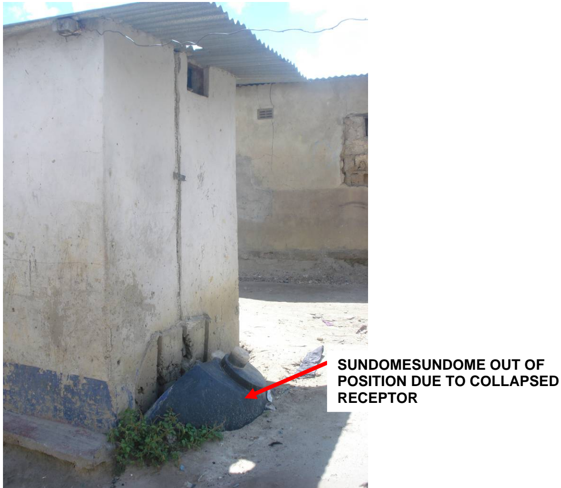
Figure 7.5: Sundome out of position due to collapsed receptor
