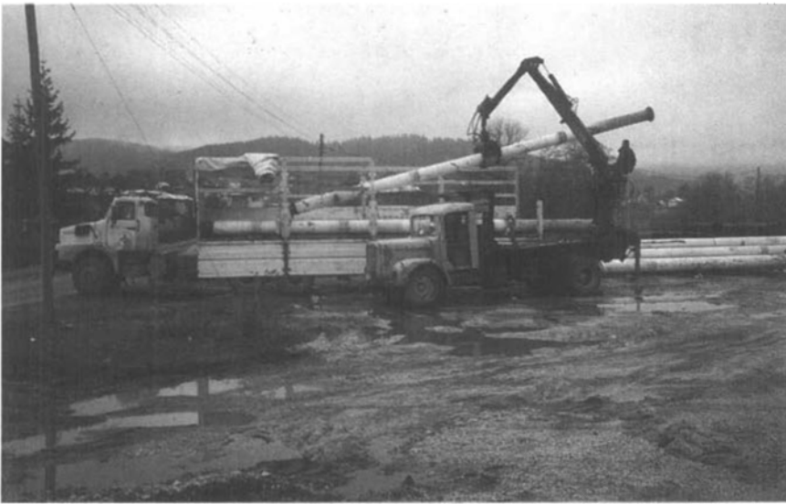
Finding a crane that was normally used to load pine logs to shift the pipes was a real coup!
