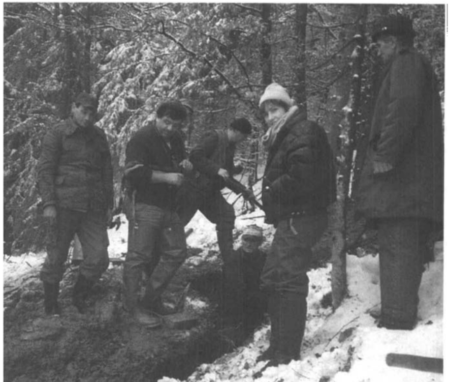
Repairing the main pipeline to Sarajevo in the snowy mountains outside Pale.
