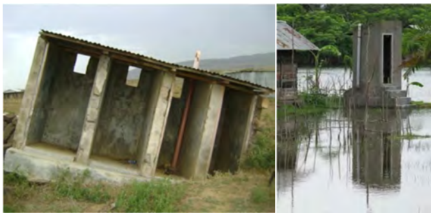
Figure 6 A collapsed pit latrine after rains in Narok, Kenya on the left and a UDDT withstanding a flooding in Bangladesh (photo by P. Mboya, 2008 and A. Delepiere, 2009)
