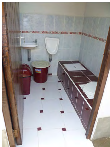
Figure 26 UDDT with barrierless ground level entry. Though not designed for people with disabilities it can be easily modified with handrails and bars (photo by H. Hoffman, 2011)
