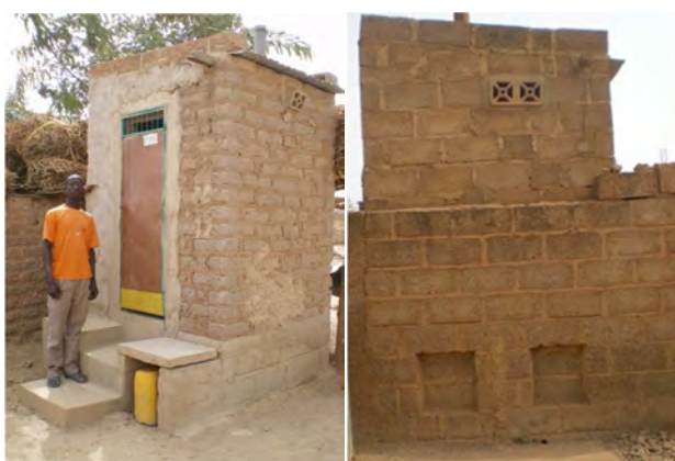
Figure 2 UDDT outhouse in Burkina frontview and rearview with faeces vault doors (photo by A. Fall and S. Tapsoba) 6
