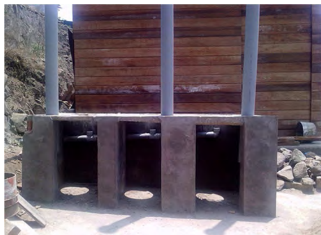
Figure 20. Plastic urine piping with slope and diameter of 5cm visible inside the vaults, Peru (photo by H.Hoffman, 2009)
