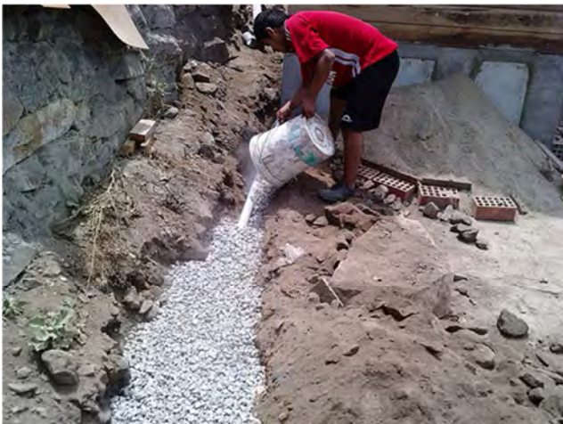
Figure 31. Infiltration trench for greywater and urine at a school in Peru (photo by H. Hoffmann, 2009)
