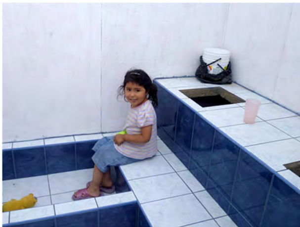
Figure 24. Bench UDDT with an attached shower under construction in San Juan de Miraflores, Peru (photo by H. Hoffmann, 2011)
