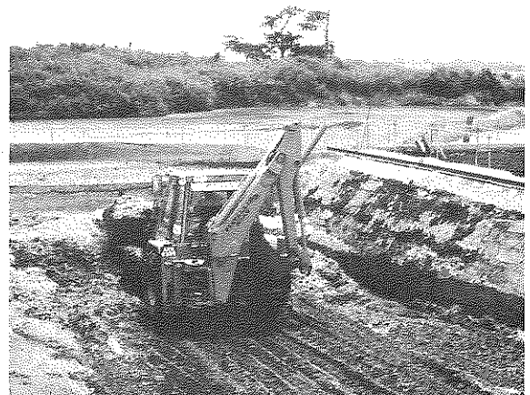
Photo 3: Sludge removal by front-end loader from a batch-operated settling/thickening tank. Achimota FSTP, Accra (Ghana).
