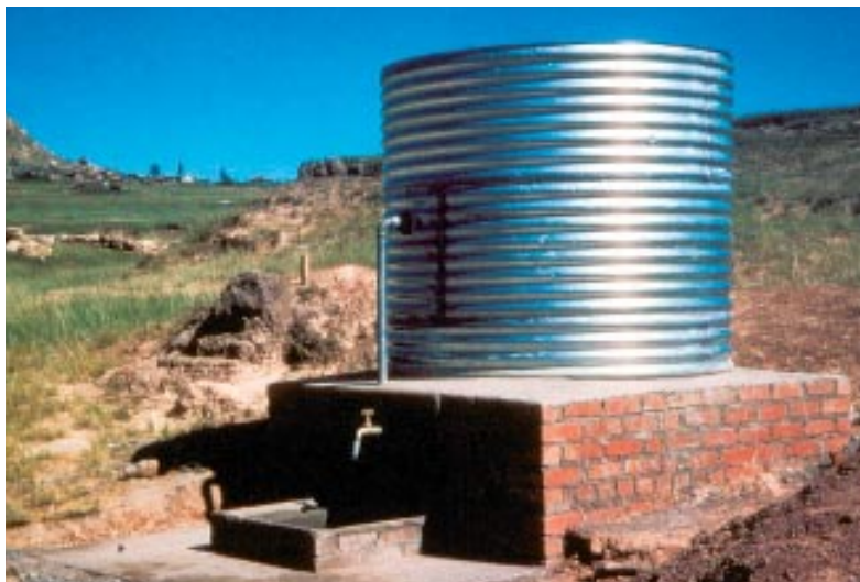
A galvanized tank for emergency water supply.
