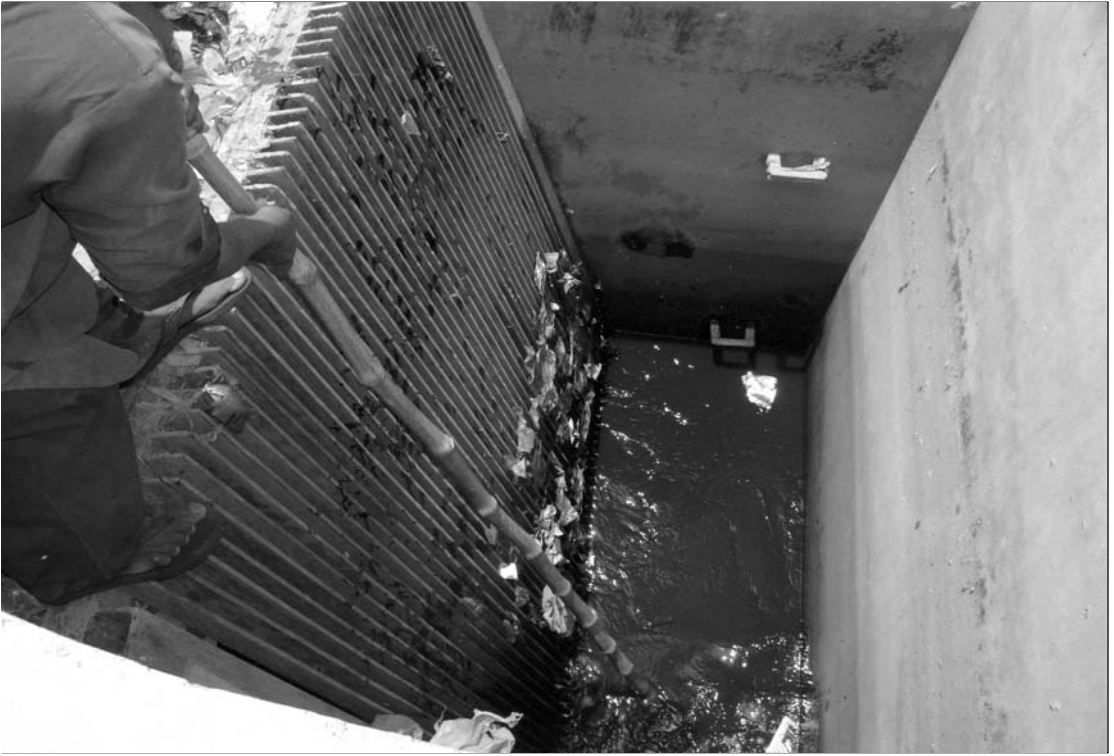
This shows the screen chamber on the inlet to the pumping station, Daska, Pakistan. The incoming sewer is surcharged and the resulting reduced flow velocity will lead to silting in the sewer.
