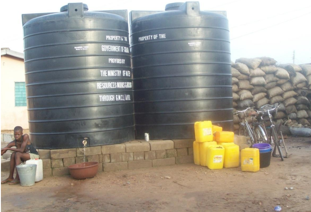
Picture 1: Water Tankers installed by AVRL at a selling points
