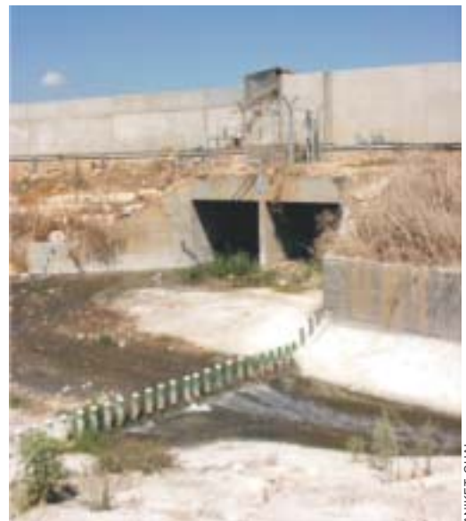
Untreated wastewater from Tulkarm is deviated into an Israeli emergency treatment plant to prevent pollution to the Alexander River downstream.
