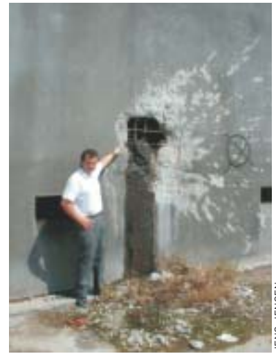
Damage sustained to the wastewater treatment plant in Gaza from Israeli military action
