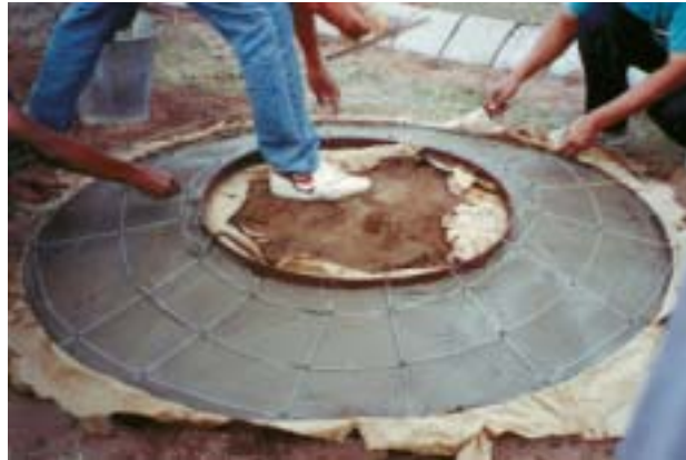
Figure 3-22: Make the lower cover wire reinforcement and two handles on top of the conical sand base. Use 0.3 centimetre diameter binding wire for reinforcement and 0.9 centimetre diameter iron bar for handles. The arrangement of handles and binding wire reinforcement is shown in the photo.
