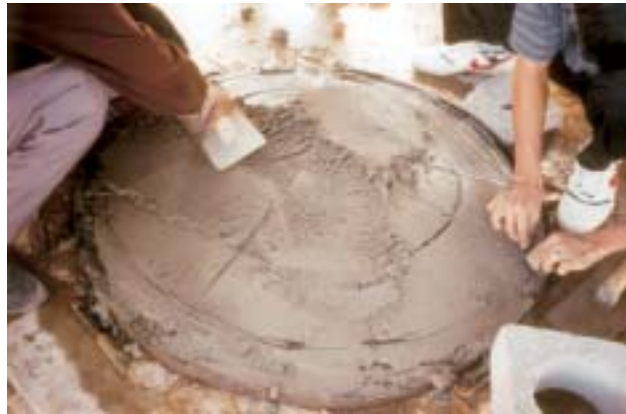
Figure 3-19: Add another layer of the 1:2 cement mortar mixture on top of the wire reinforcement; fill up to the top level of mould. Remove the outer mould after one hour, before the concrete mortar is set. Cure the cast upper cover with water for at least 3 days, though, again, curing for 7 days is better.
