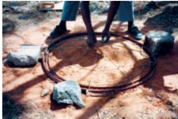
Figure 3-15: Make the upper cover wire reinforcement and two handles on top of the conical sand base. The 0.3 centimetre diameter binding wire is used to make the reinforcement and 0.9 centimetre diameter iron bar is used for the handles. The arrangement of wire reinforcement and handles is shown in the picture.
