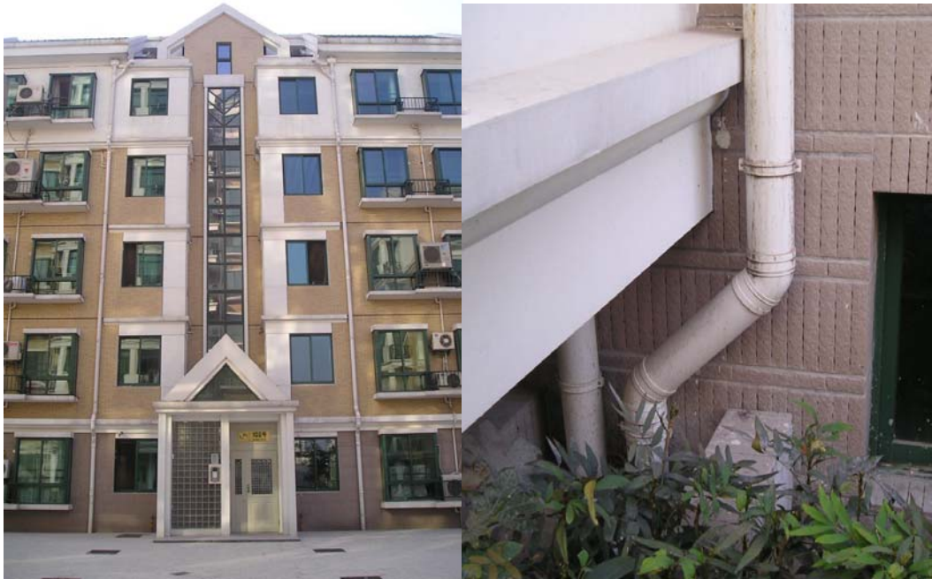
Figure 4-27: The storm water collection pipes for roofs in Nanjing Wanfuyuan Community
