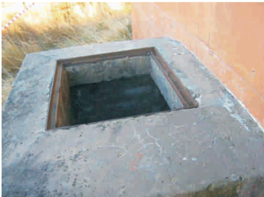
Figure 22 a,b,c: Toilet facilities in many schools are unusable due to poor maintenance, vandalism and inappropriate usage
