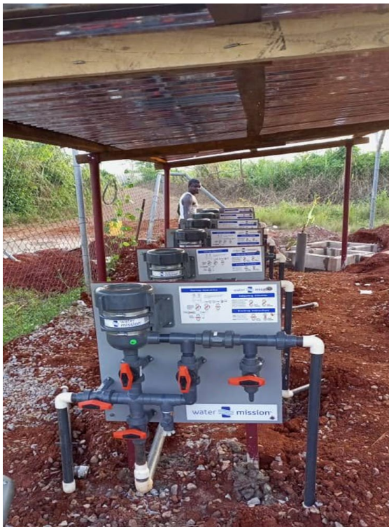
One of the technologies used as part of chlorination pilot
