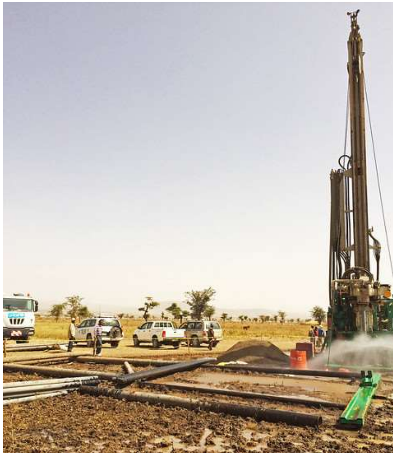
Deep well drilling in Welenchiti town in Boset Woreda of Oromia region.
