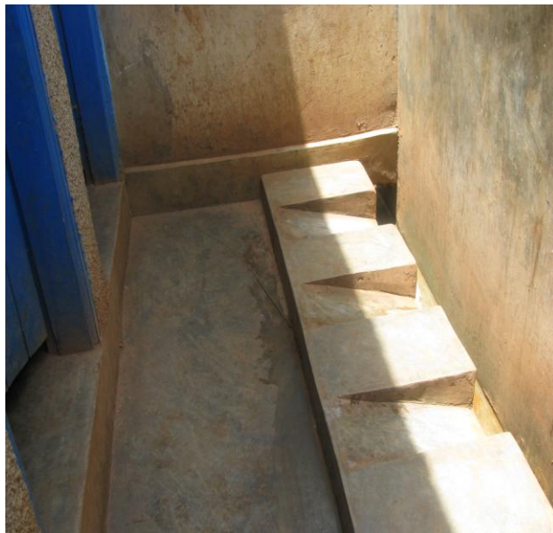
Girls' urinals at Mirembe Infant School: the urinals are constructed with a slope to allow for easy flow of urine
