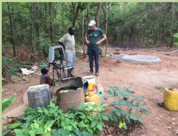
Figure (above) manually drilled borehole and rope pump, plus recharge well with well owner and Rik Haanen of Jacana Zambia (photo: Sally Sutton)
