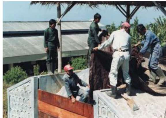
Covering work of plastic sheets (A roof is put up using coconut leaves to shut off the direct sunlight.)
