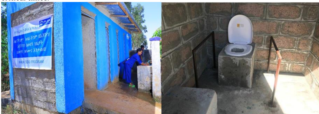
Figure 5: Disability inclusive school WASH facilities, Bahir Dar Zuria and Last Districts Photo credit: Plan International
