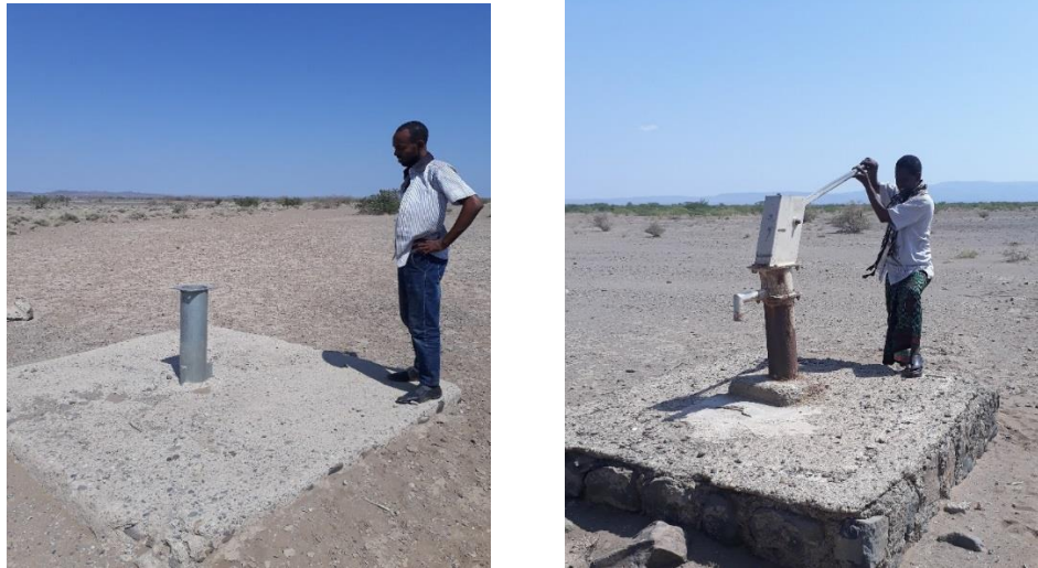
Picture 7. The two non-functional pumps in Amestegna village
