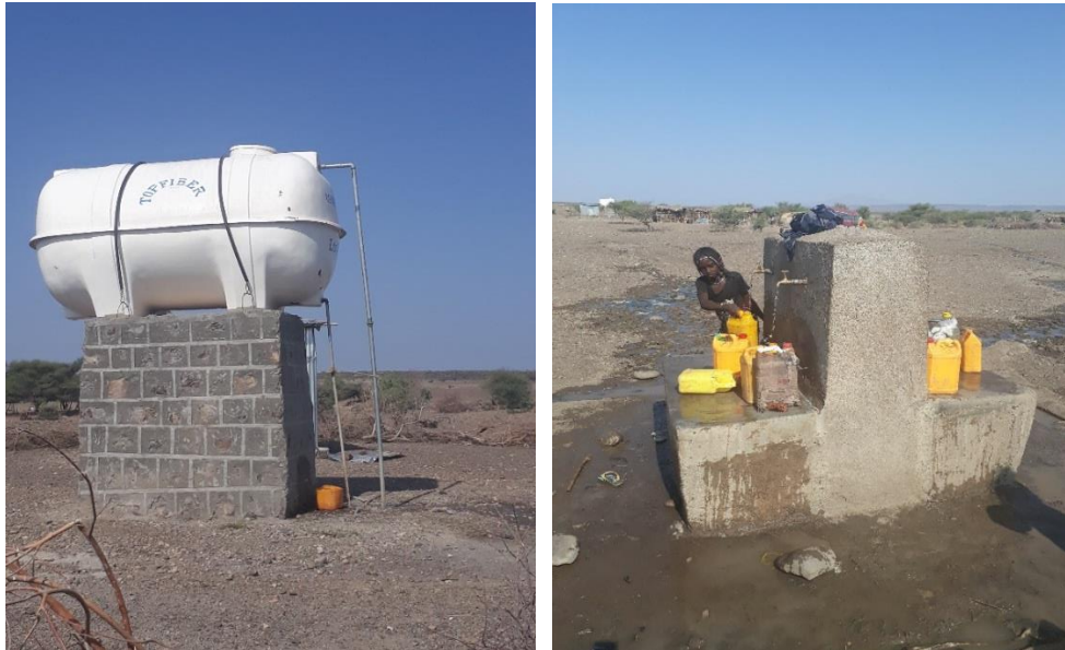
Picture 10- Motorized water pump with stand pipes in Wayta lete village
