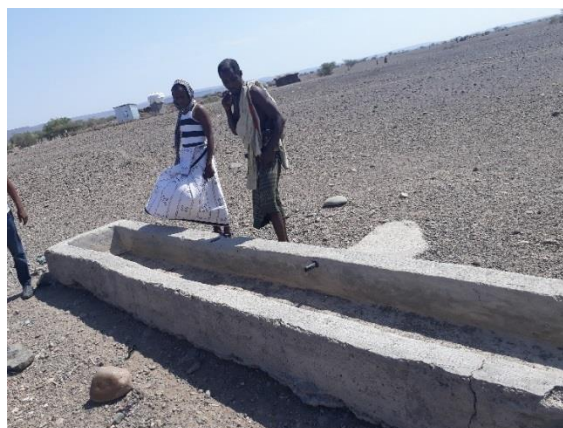
Picture 11 Cracked water trough in Wayta leta village
